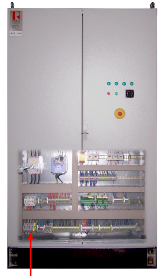
Supply terminal block
